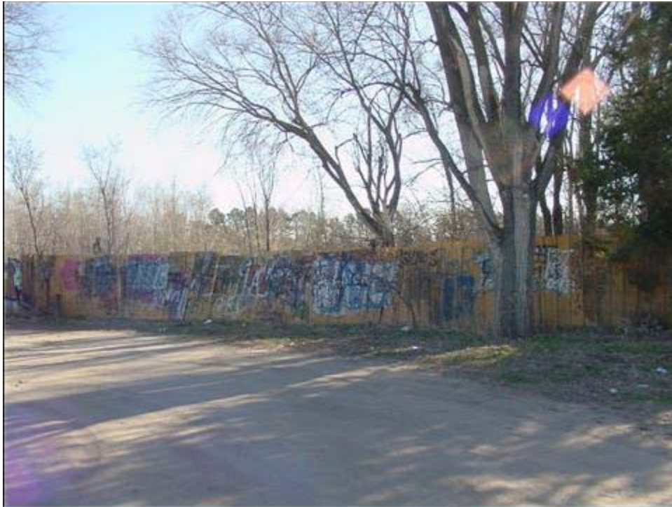
Photo E-42. Vandalism at Tailrace Park: photographed April 5, 2011.
