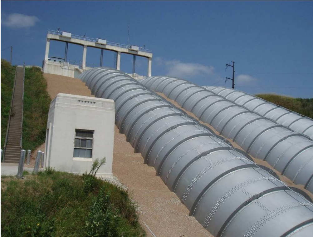
Photo E-20. View of the Penstocks from the Columbus Powerhouse.
