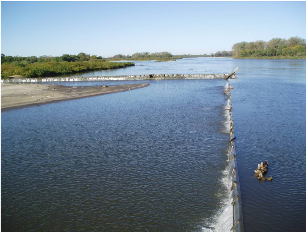
Photo E-2. View of the Diversion Weir from the Sluice Gate Structure.
