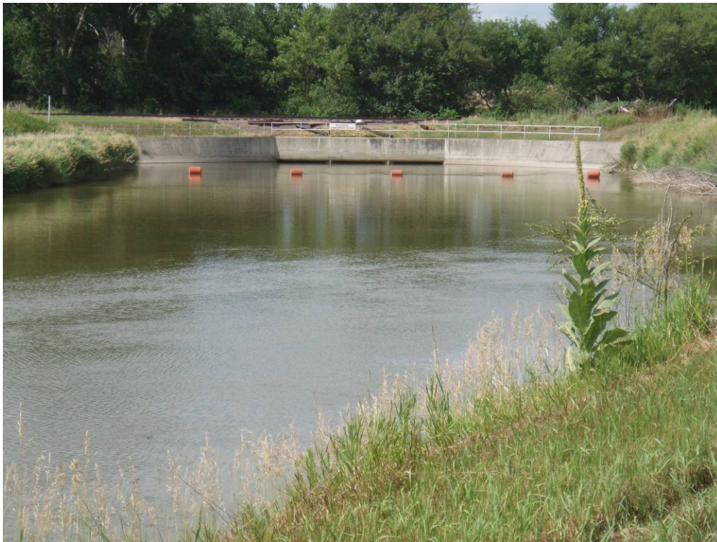
Photo E-10. View of Upper Power Canal and the Railroad Siphon at Genoa.
