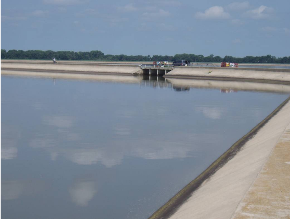
Photo E-17. View from Lake Babcock to Lake North showing the dike that divides the two regulating reservoirs and the control structure that connects them.
