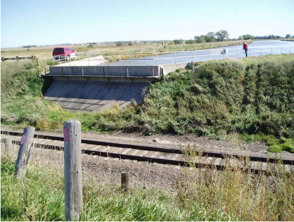
Photo E-14. View of the Lower Power Canal at the Oconee Siphon exit.
