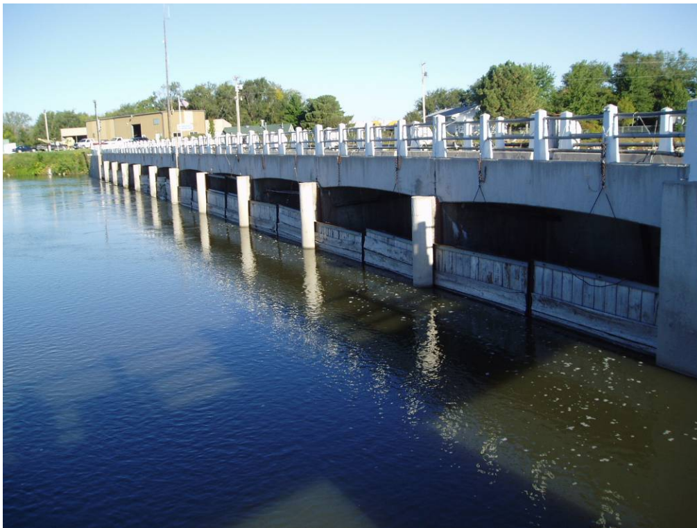
Photo E-3. View of the Intake Gate Structure from the Sluice Gate Structure.
