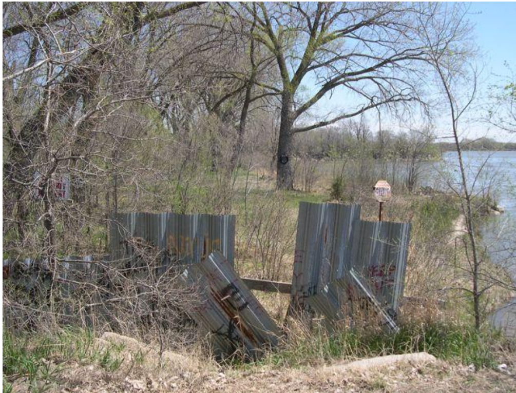
Photo 9. Vandalism at Tailrace Park.
