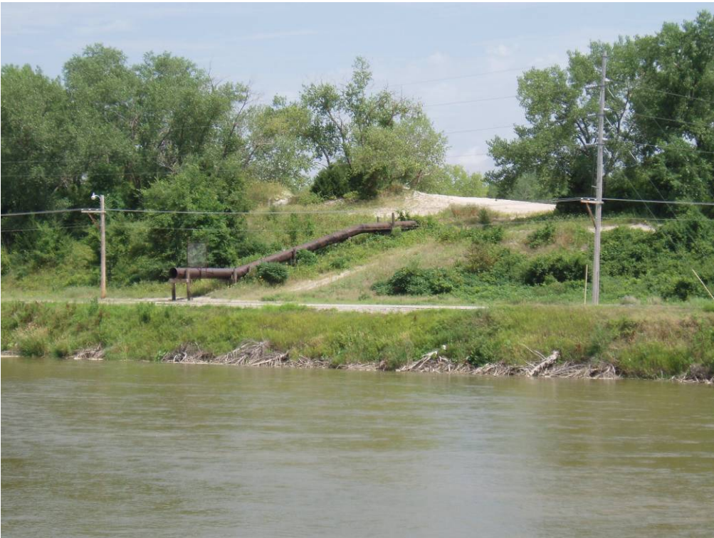
Photo 4-12. Typical discharge piping and shoreline stabilization at the South Sand Management Area.
