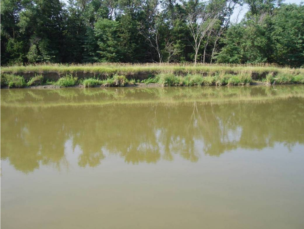
Photo 5-1. An undermined slope on the Lower Power Canal.
